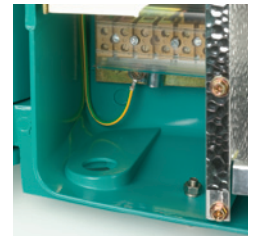
Cable entry and termination block
